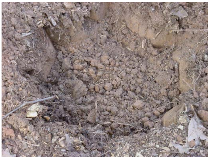
Hand dug planting hole with notched walls to enhance root spread into the surrounding clay soil.
